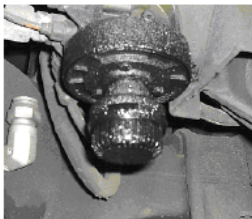
Air dryer exhaust with oil present
